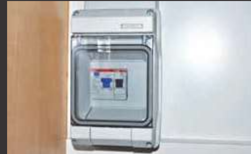
Distribution box with RCD and fuse (16 A)
